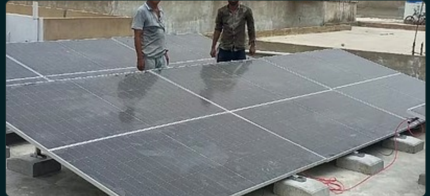
ROOFTOP SOLAR INSTALLATION — KARACHI
